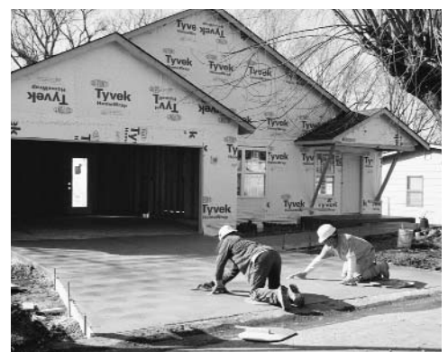
Work is progressing on the HBA-sponsored Habitat House in Wentzville for a family victimized by Hurricane Katrina.
