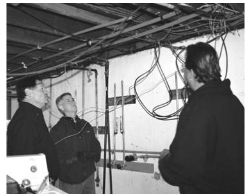
Project manager and HBA builder member Dennis Boxdorfer of Denco Construction Services (left) checked the wiring with HBA associate member Gus Catanzaro of J-Mar Plumbing and Steve Miller of Denco Construction Services .
